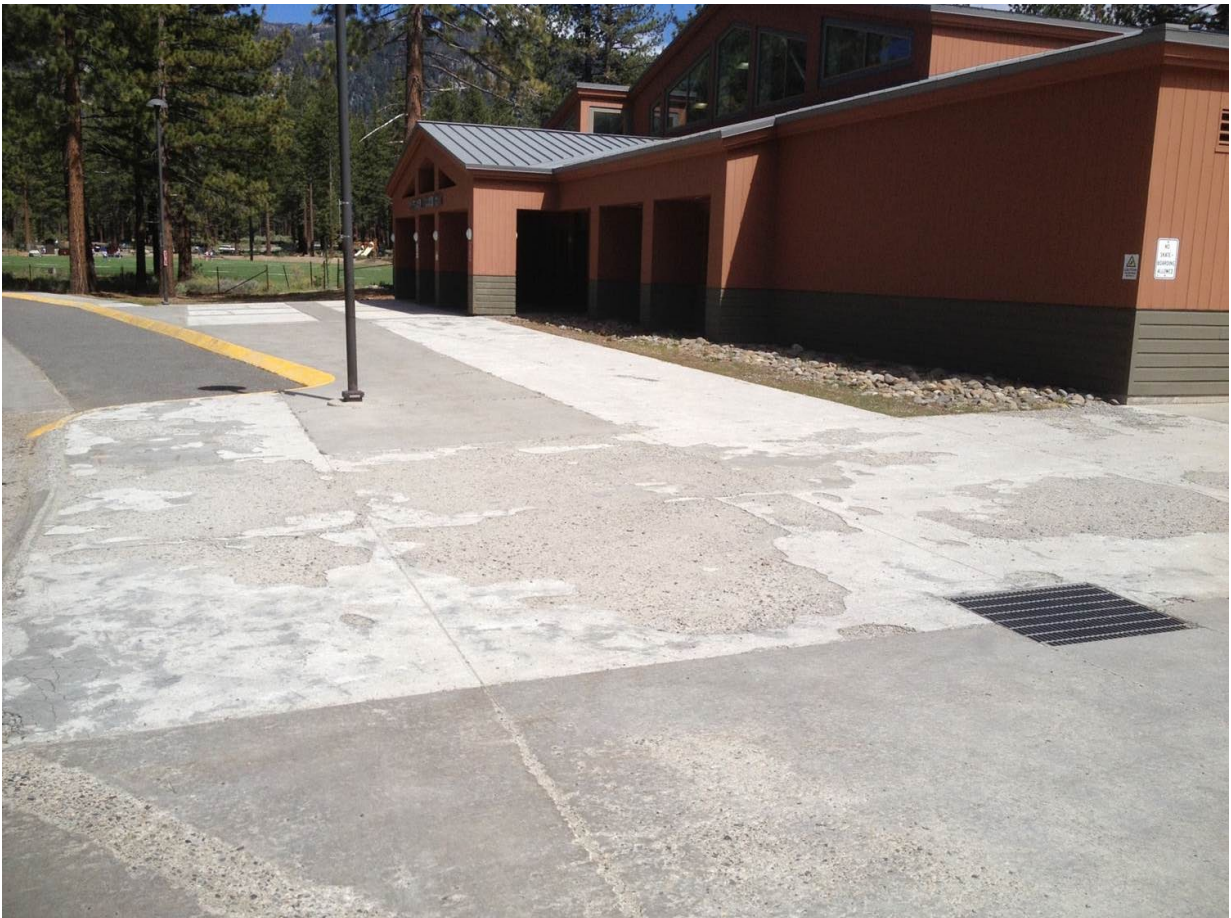
Concrete Deterioration in Front of Physical Education Center
