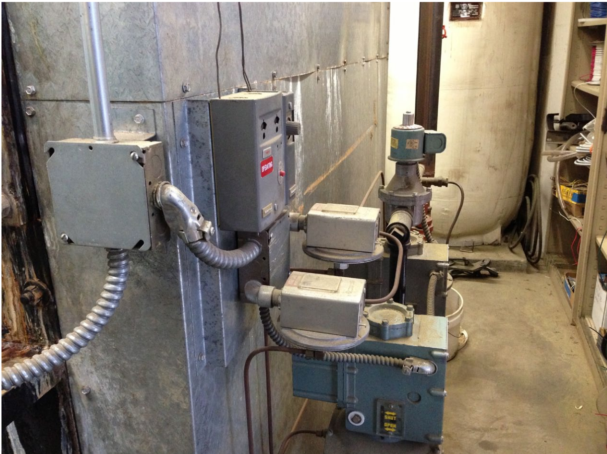
Aged HVAC Equipment
