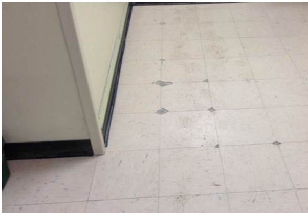
Typical Flooring Deterioration
