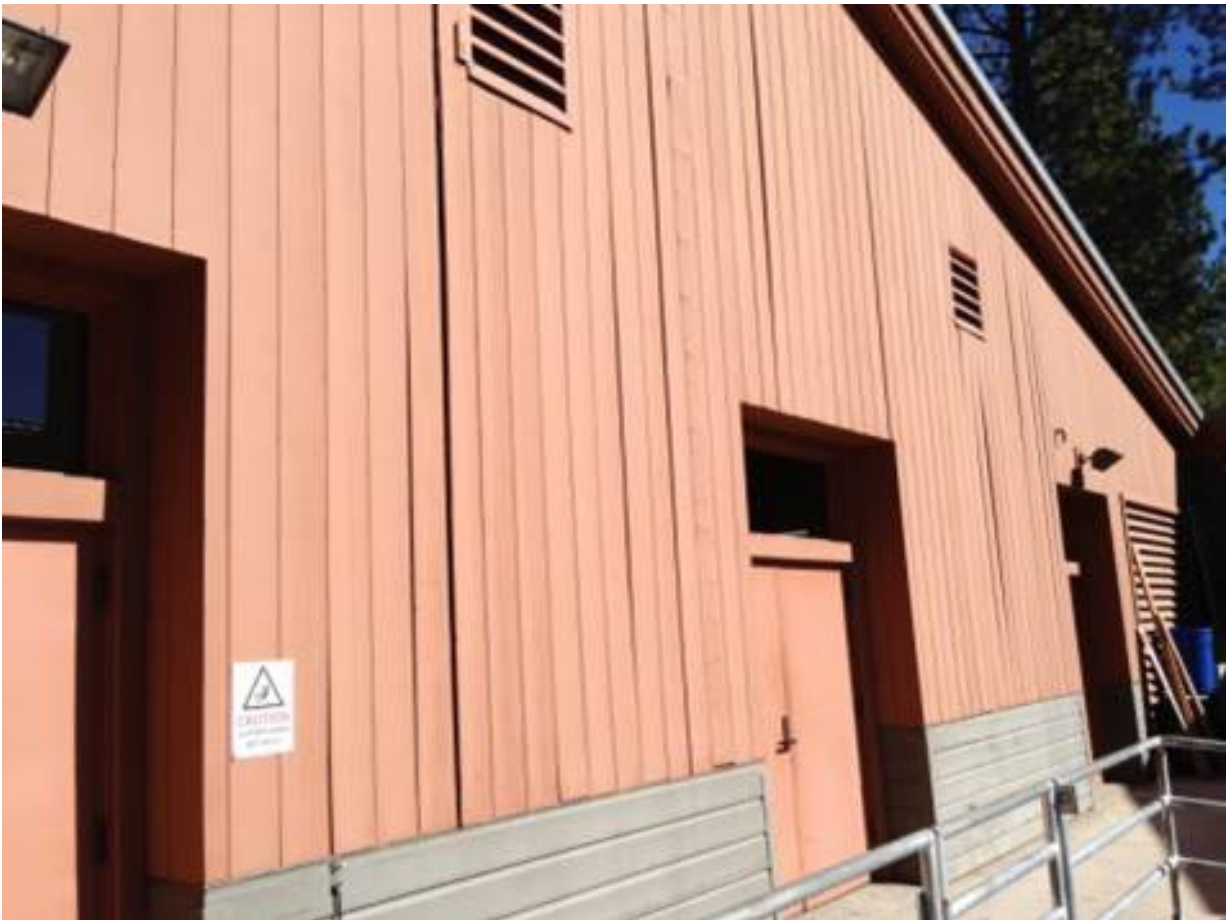
Typical Exterior Wood Siding Bowing and Separation
