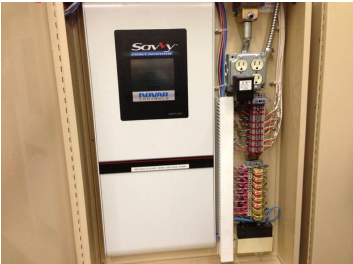
Outdated Energy Management System
